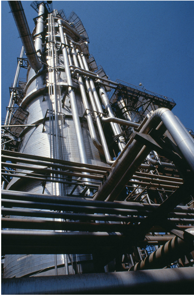
Ras Tanura Refinery (Used with permission from Houssain Ramadan/ Saudi Aramco World/PADIA )
